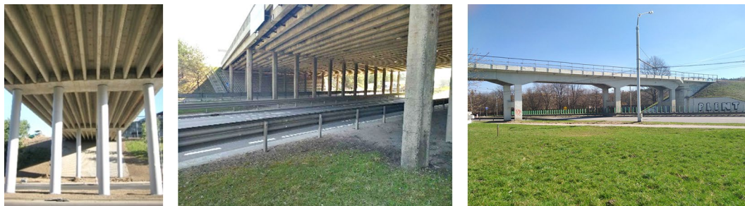
Fig. 2. The transport industry structures operating in highly aggressive media
