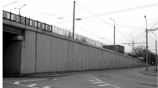
Fig. 1. The general view of the auto-road overpass and the strengthening fencing structures
