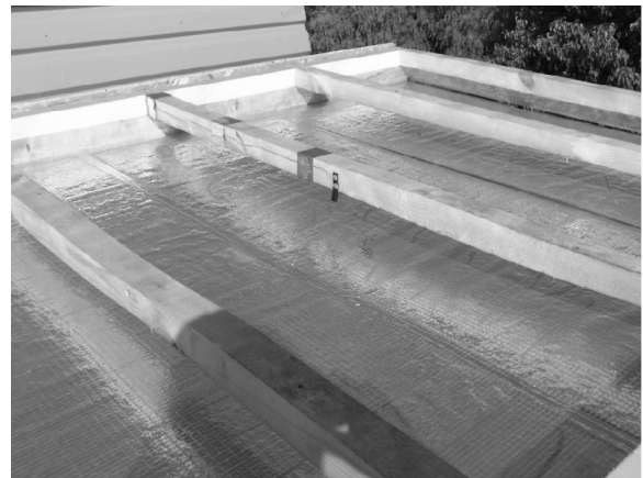
Fig. 5. The mounting of the cement-sawdust board with heat reflective coating in cell S2 (exp. No. 3)
