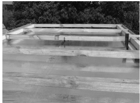
Fig. 7. The mounting of the two air gaps, separated by a heat reflective coating with two heat reflecting surfaces, in cell S2 (exp. No. 5)
