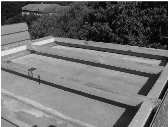
Fig. 6. The mounting of the cement-sawdust board without additional coatings in cell S2 (exp. No. 4)
