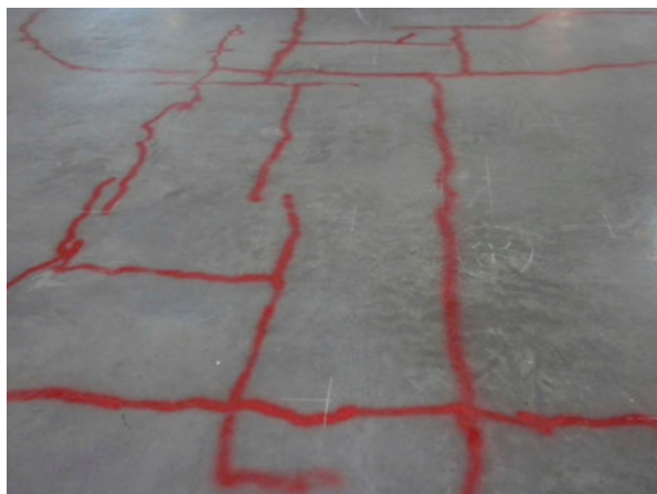
Fig. 5. View of the situation of cracks in concrete floor slab
