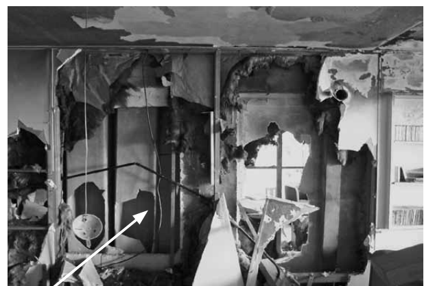
b) Damaged vertical ducts
